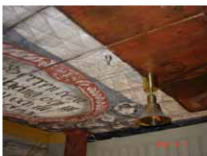
An automatic high-pressure water mist nozzle in Älgårds church. The position of a nozzle is often a compromise between fire protection, cultural historical and aesthetic demands. (An overview of fire protection of Swedish wooden churches, Magnus Arvidson, Brandforsk project 500-061 http://www.brandforsk.se/MediaBinaryLoader.axd?MediaArchive_FileID=32f260f3-64b1-4f83-9442-ad1a5eed6097&MediaArchive_ForceDownload=true )
