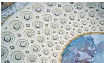
The dome of the US Library of Congress – spot the sprinkler! ( http://www.buildingconservation.com/articles/firesup/firesup.htm )
